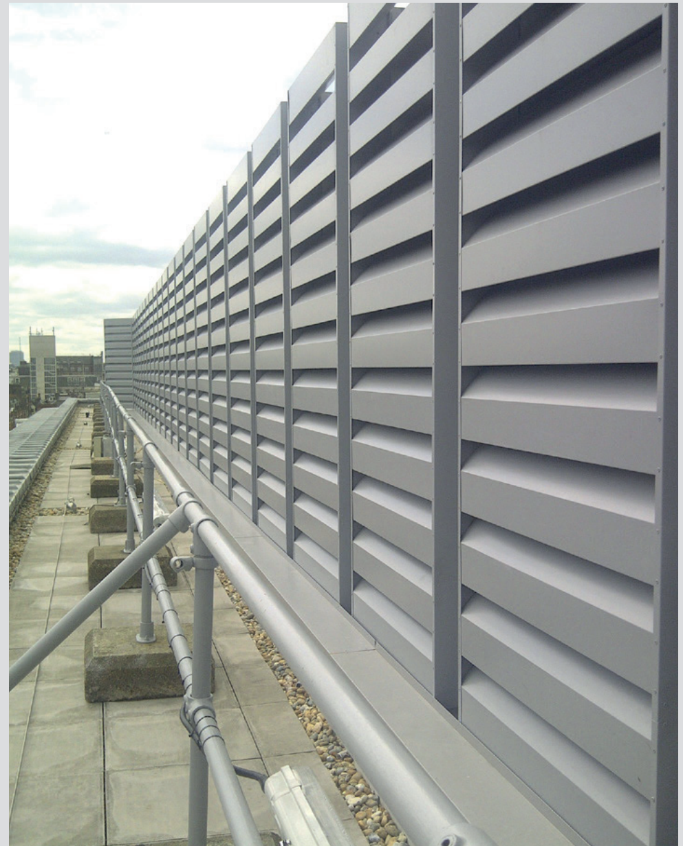
Right: Great Portland Street, London. Acoustic louvre.
