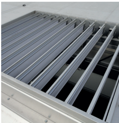
Seefire as termination piece above a fan (guard removed)
